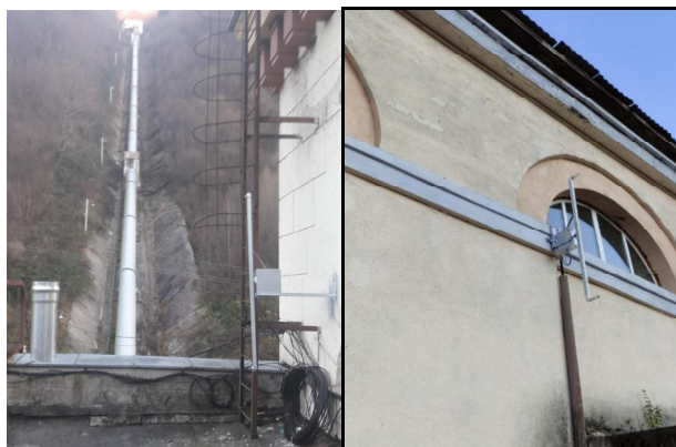
Fig. 6. Meteorological stations with a temperature gradient installed on the generator hall (left) and on the throttle gate building (right)
