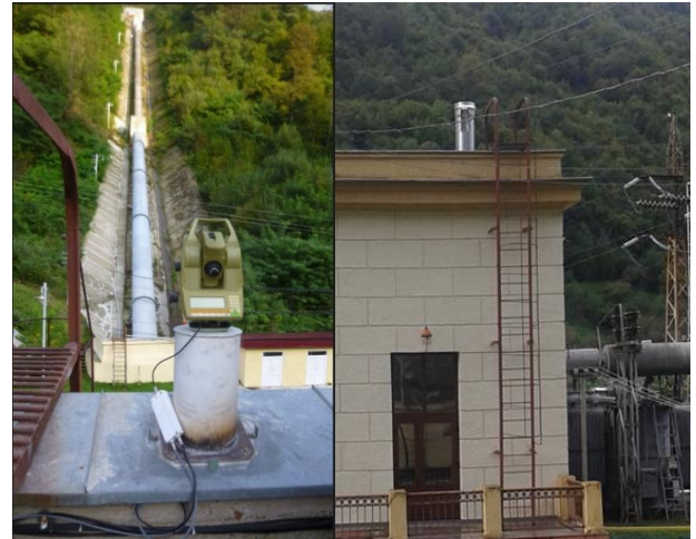
Fig. 4. Robotic total station LEICA TPS1000 with thermal protection installed on the roof of the generator hall
