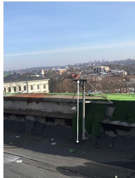
Fig. 9. The height component of the marked points survey site in Geoterrace ( h=150 cm)
