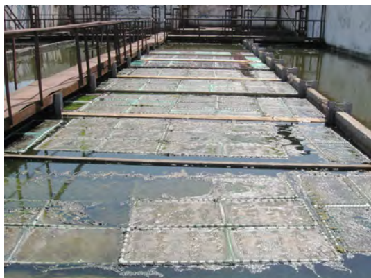
Fig. 3. 76 rafts with fiber carrier “VIYA” installed in the experimental section of the sewage treatment plant of Motor Sich JSC in 2017
