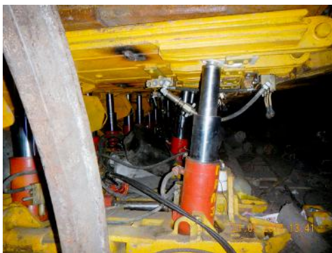
Fig. 7. State of the powered support of the coal extracting complex
