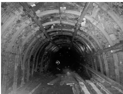
Fig. 8. State of the extraction mine working in M. I. Stashkova Mine (Western Donbas)
