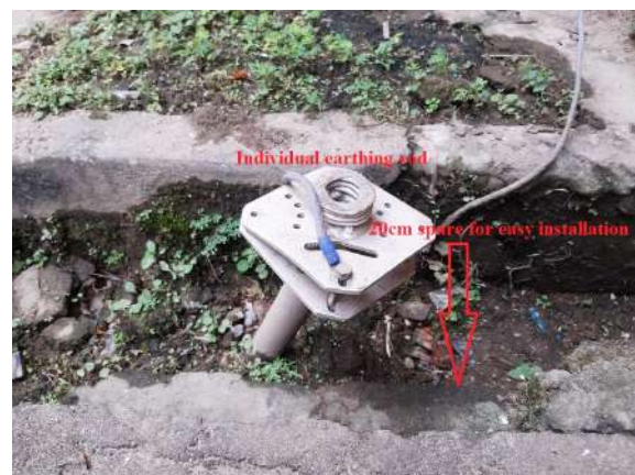
Fig. 3. Individual earthing rod that is wired to the motor frame with 20 cm spare length for easy installation
