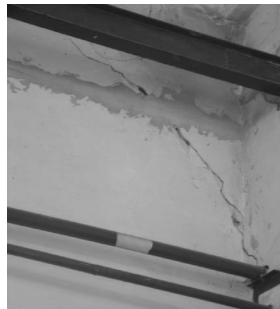
Photo 6. Vertical crack of the wall at the crossing of axis "3"... "B"
