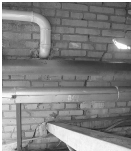
Photo 5. Vertical crack of the wall along axis "3" between axis "A"... "B"
