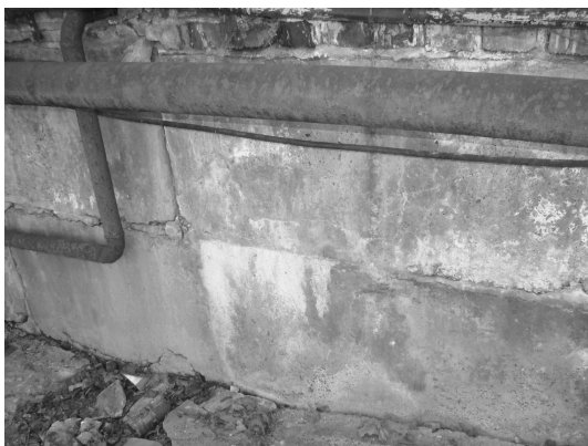
Photo 3. The state of the foundation of wall blocks by axis "B" between axes "1/1" ... "3". Moving units by horizontal and vertical seams and by contact of walls and blocks
