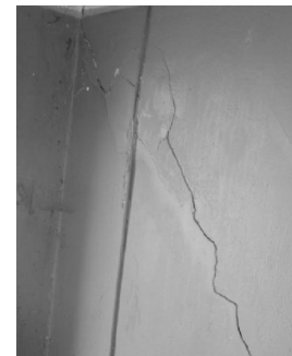
Photo 8. Vertical crack of the wall on the second floor at the crossing of axis "A"... "1/1"
