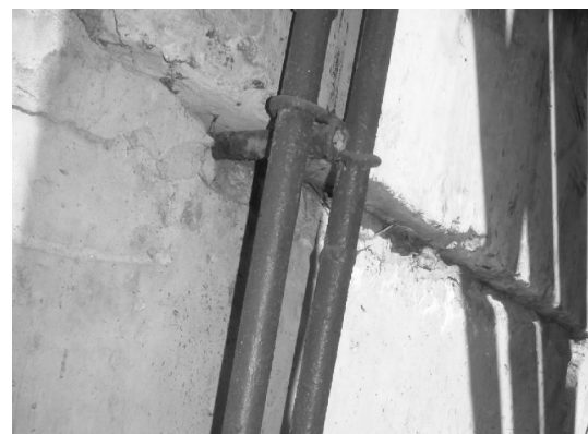
Photo 4. The state of the foundation wall blocks by axis "A" between axes "2" ... "3". Deviation from vertical, moving units by seams
