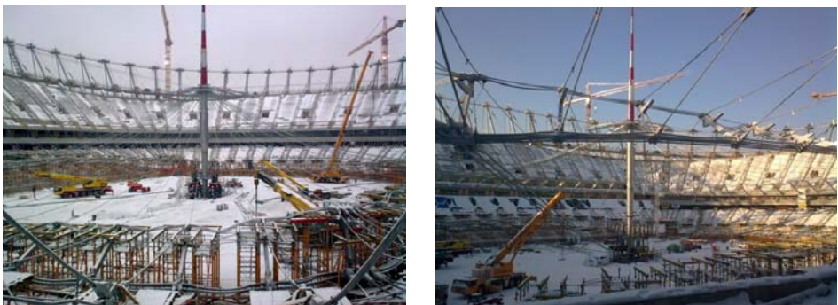
Fig. 10. Connection of lines of the permanent and foldable roof and tensioning of the lines, two rings with spreaders and three lines for suspension of the mast
