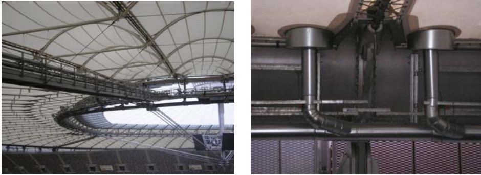
Fig. 15. One of the suspended bridges leading to the circumferential pavement with water gutters; permanent roof drainage in the vicinity of the main junction of the compressed ring with the pole and tensioning string
