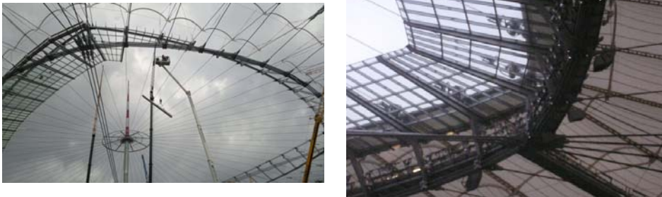
Fig. 12. Assembly of the glass roof brackets; above the glass roof there are visible lines of the foldable roof and anchoring elements; under the lower ring there is a visible connection of bearing strings with the strings, which suspend the mast
