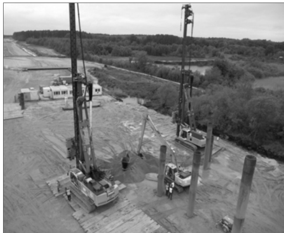
Figure 7 – Two heavy Liebherr rams during installation of geotextile encased columns, standing on wooden platform placed on already installed GECs
