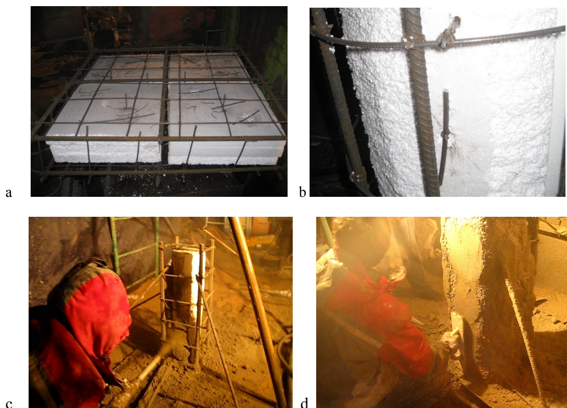
Fig. 1. Production of fragments of reinforced concrete structures: a – a metal frame with a non-removable liner; b – fixing of the liner made of polystyrene; c – spraying of the square pillar fragment; d) surface smoothing after wet spraying
