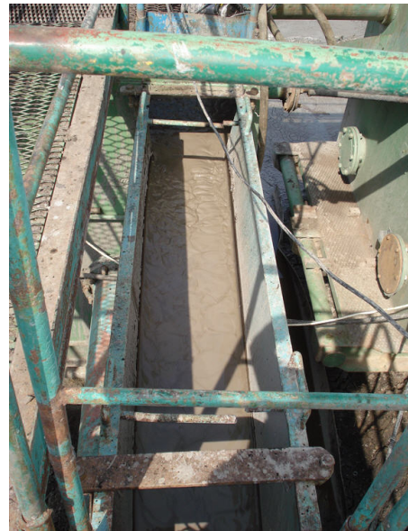
Figure 1. Unsealed channels of a pumping-circulatory system
