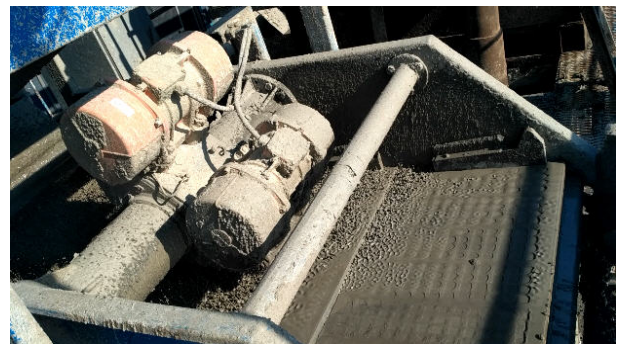
Figure 5. Mud screen in the operating mode
