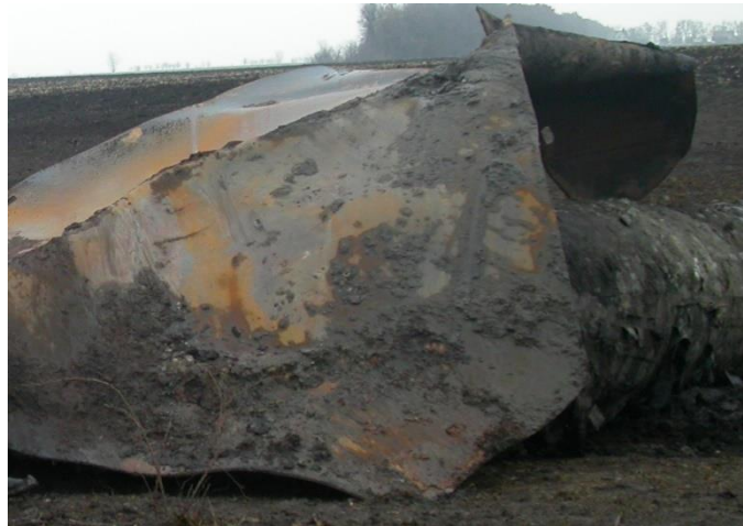
Figure 1. A typical example of a catastrophic destruction of the 1420 mm diameter pipe of the main gas pipeline Urengoy-Pomary-Uzhorod (2007 near the compression station Ilyinty)
