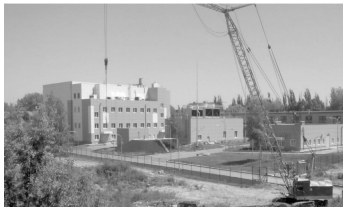
Fig. 7. The building of the Neutron Source Facility under construction in Kharkiv (© SSTC)
